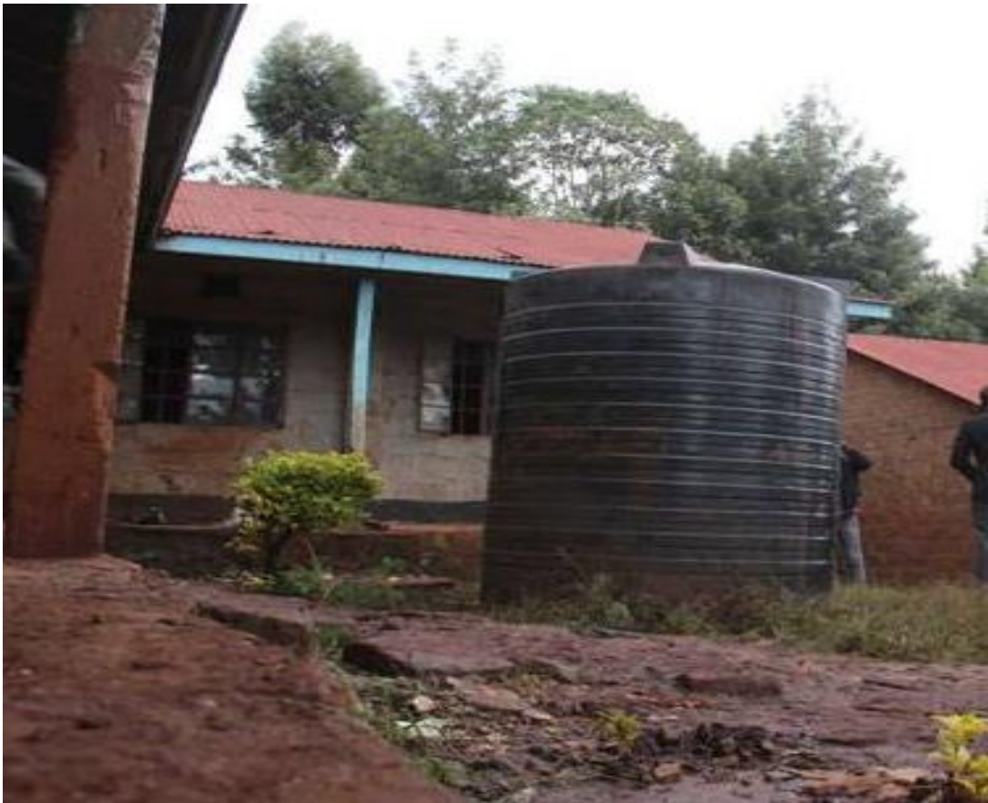
1. A water storage tank used in a school
