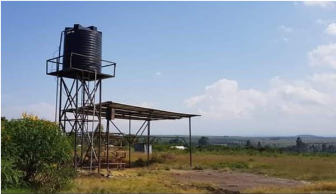
Figure 5: Water storage tank in one of the Community Conservancies\
