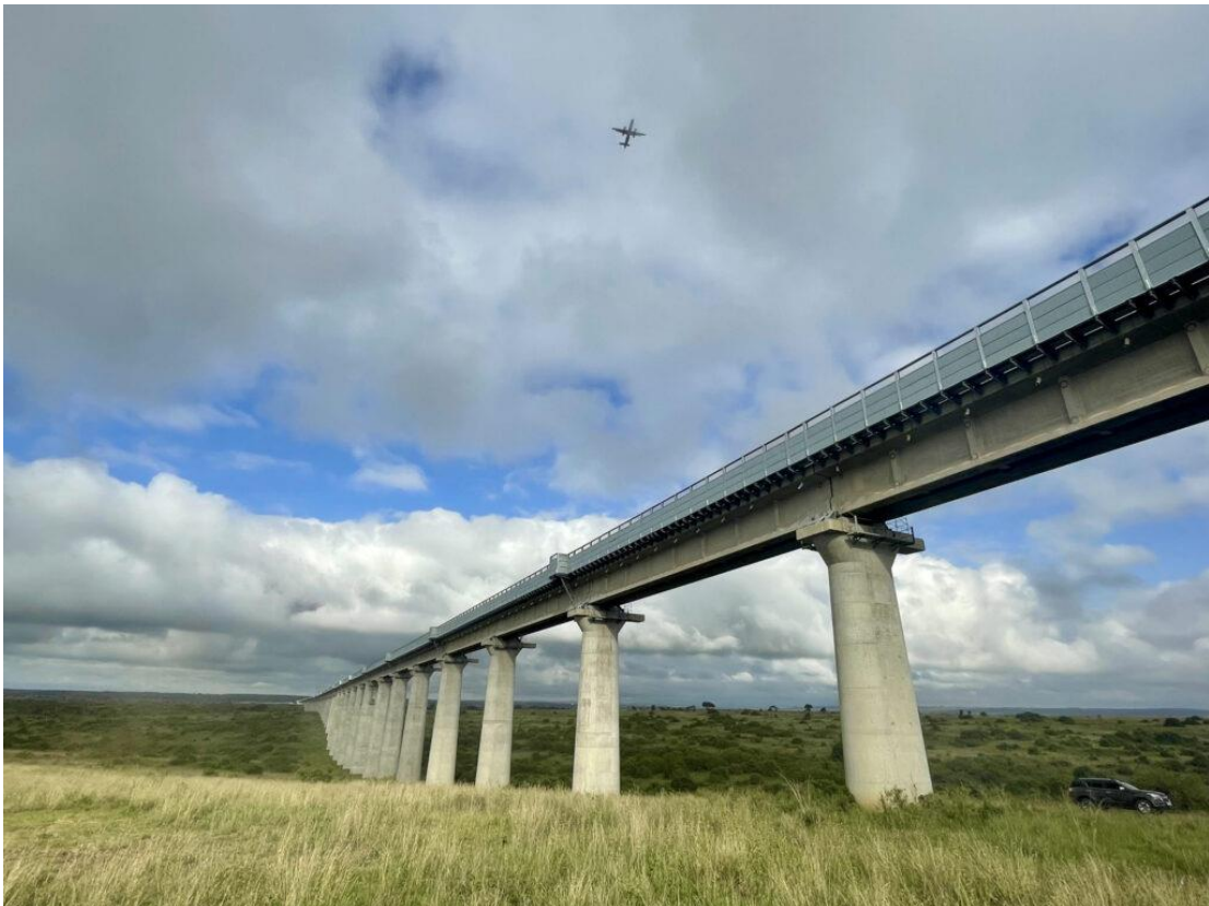
Plate 2: The SGR pylons at the Tsavo River
