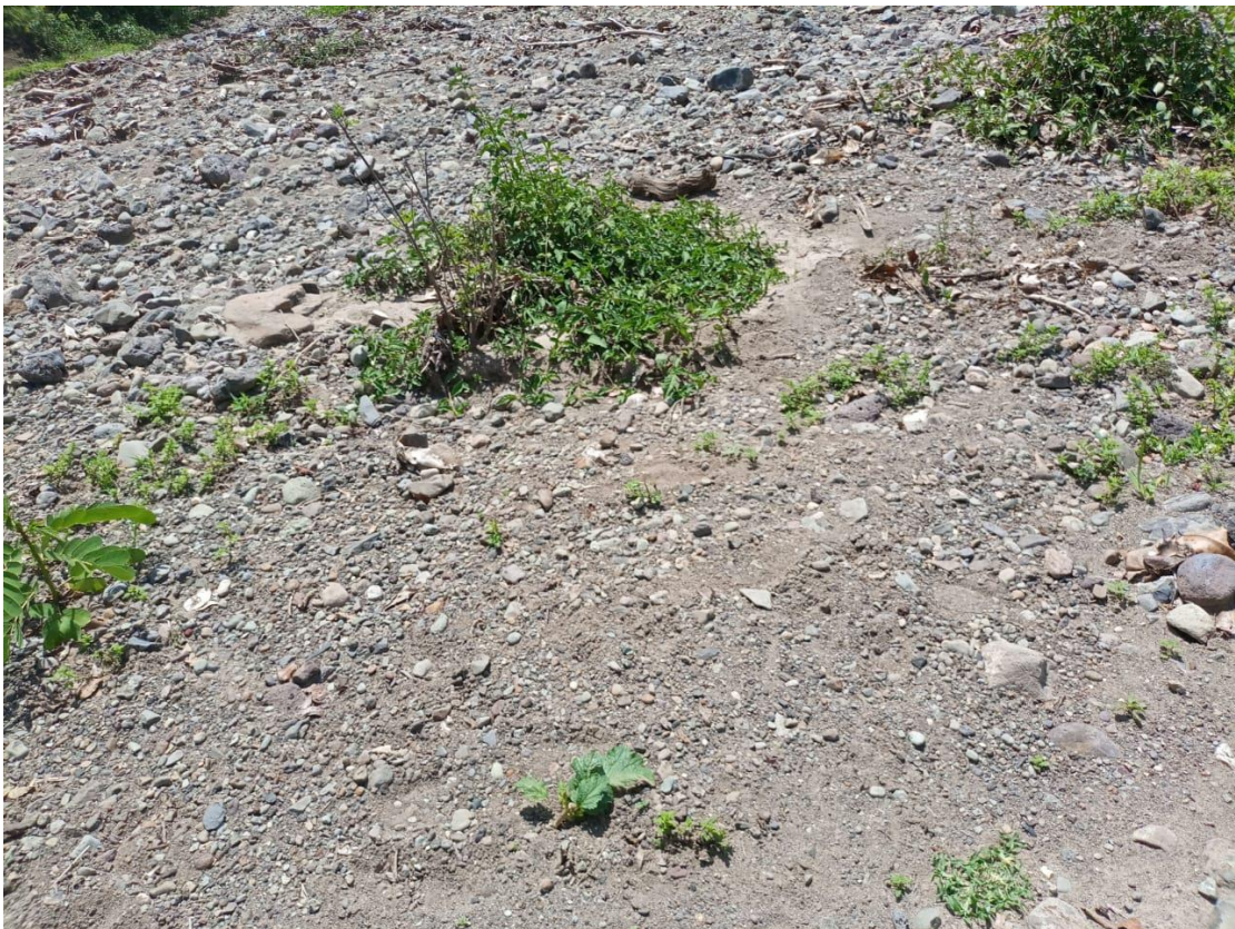
A stone mantle showing severely eroded area within the Kimao catchment
