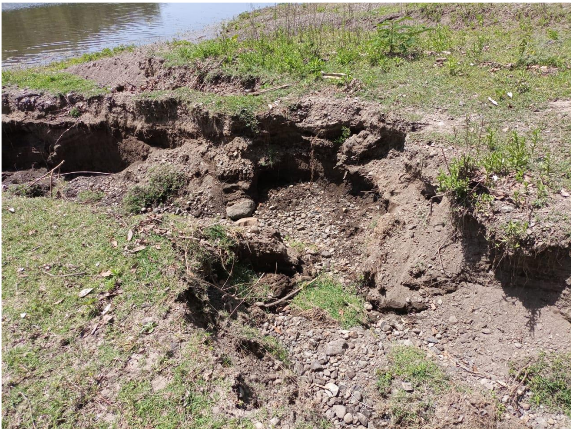
Erosion of top soil and formation of Gullies
